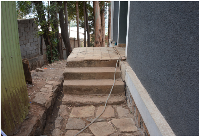
Fig. 49. Improper design. These stairs have uneven steps; there is a lack of handrails on both sides, and no visual contrast, posing a safety hazard for people with balance, mobility, and visual impairments.
