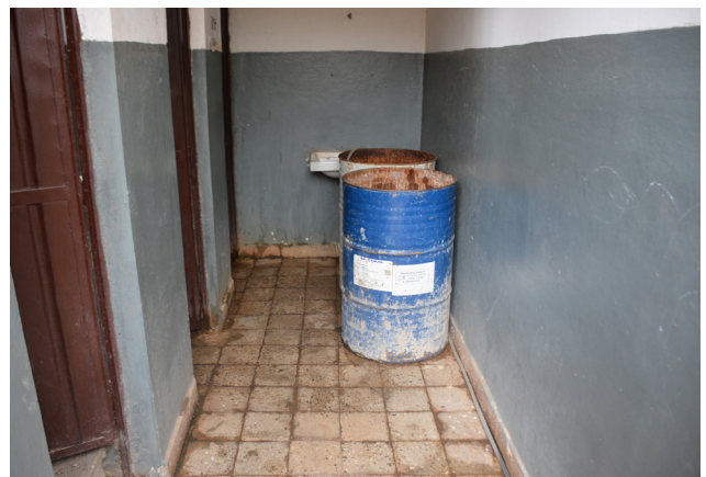
Fig. 82. Misuse of space. The path to the accessible toilet is blocked by obstructing objects, making it impossible for people with mobility aids to access it.
