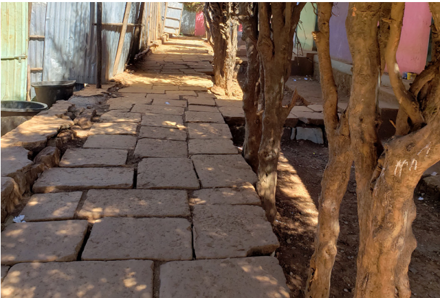
Fig. 28. Uneven pathway. Uneven surfaces and wide gaps on the pathway create risks of falling, tripping, or getting stuck, particularly for people using mobility aids, crutches, and white canes.
