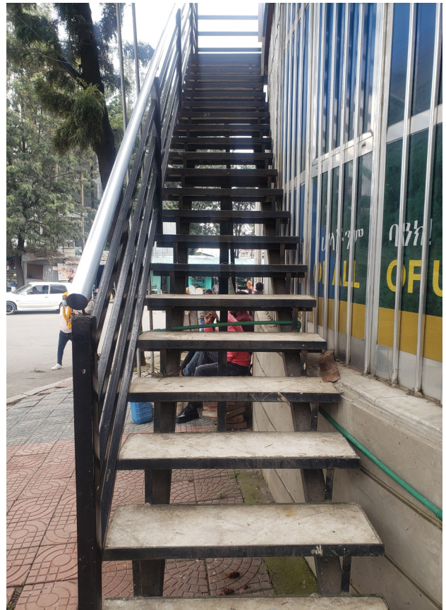
Fig. 51. Steep staircase with open risers. Open risers should be avoided as the empty space under the steps may increase the risk of tripping and injuries. Moreover, these stairs are too steep, and there is a lack of an intermediate landing, (recommended after every 10–15 risers).
