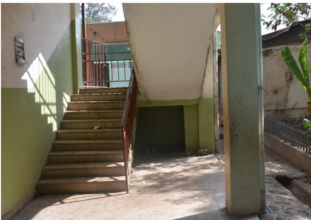
Fig. 50. Open space under the stairs. To prevent collisions or accidents, the open space under the stairs must either be closed off or have a permanent guard or protective barrier installed.
