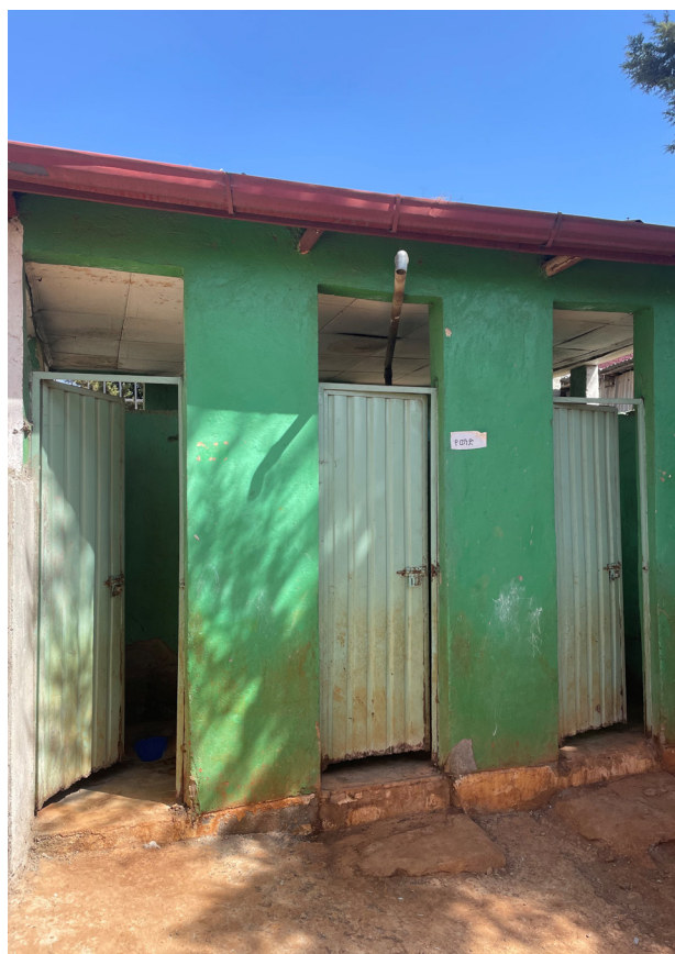
Fig. 62. Narrow doors, high threshold. These doors are inaccessible due to their narrow width (<850 mm), high threshold (>20mm), and no sufficient visual contrast between the doors and the surrounding surface.
