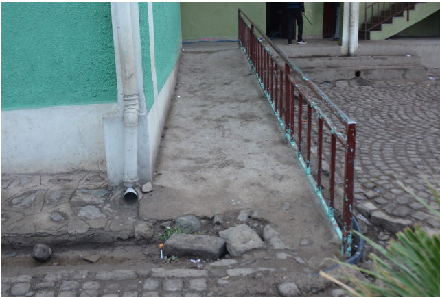
Fig. 41. Lack of maintenance. The surface of this ramp is irregular with holes and bumps, making it challenging to use with wheeled mobility aids.
