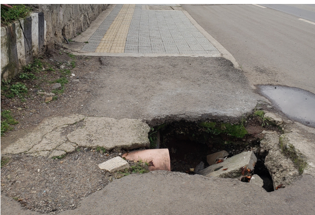
Fig. 29. Dangerous interruptions. Holes in the pathway pose a danger for everyone, particularly those with visual impairments. They create a risk of falling, tripping, or getting stuck.
