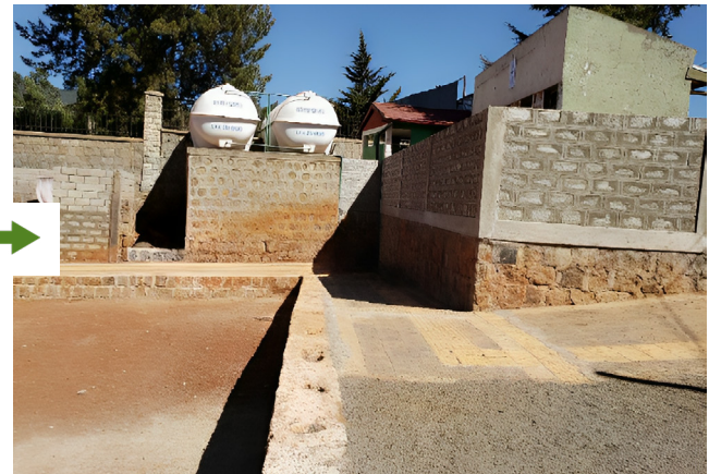
Fig 7. Circulation (after). To create safe and accessible circulation routes, a sloped pathway with tactile surfaces was constructed to connect the school's entrance to other facilities.
