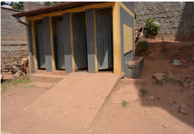
Fig. 79. Inaccessible toilet. Despite adding a ramp, the toilet remains inaccessible due to a lack of landing, narrow doors, high threshold and insufficient maneuvering space inside.
