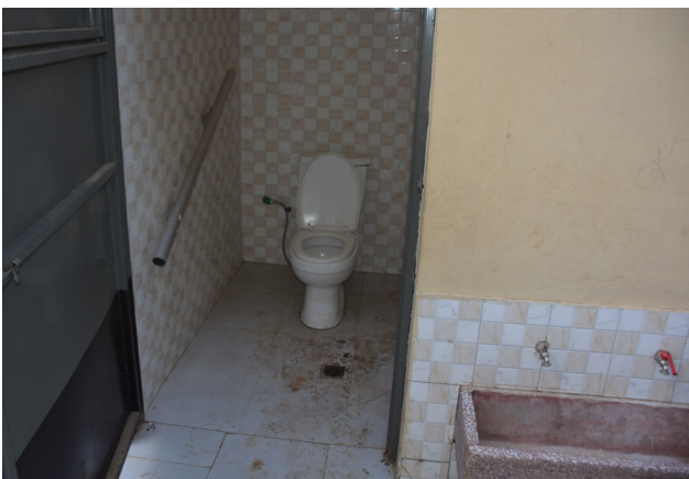
Fig. 80. Insufficient space. Despite being marked as 'Accessible,' this toilet has no sufficient maneuvering space; it lacks appropriate grab rails and accessible hand washing facilities.
