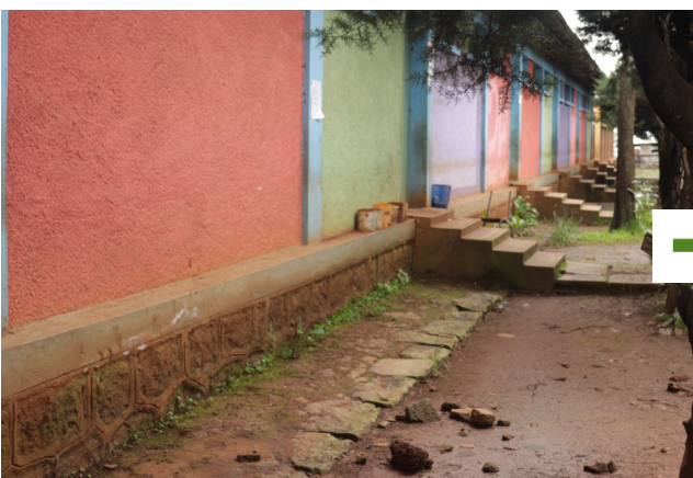
Fig. 10. Classroom entry (before). Prior to the renovation, all classroom entrances were inaccessible to different mobility aid users.
