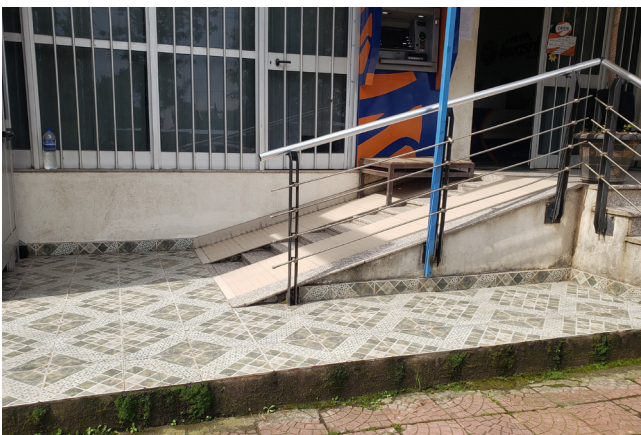
Fig. 42. Improper design. The ramp is blocked by a high curb; there are stairs positioned in the middle of the ramp; an ATM is placed on the ramp and the ramp itself is too steep. As a result, people with mobility aids are not able to use the ramp or access the area.
