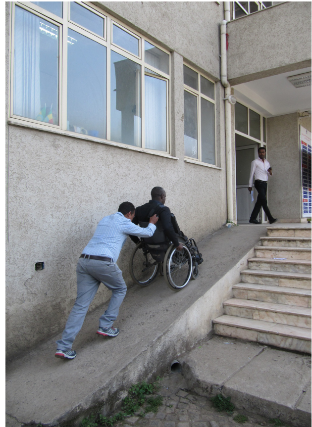
Fig. 43. Dangerous ramp. The slope of this ramp is excessively steep (>8%). The lack of handrails on either side of the ramp poses a significant safety risk for users.
