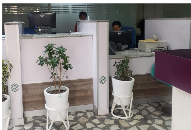
Fig. 69. Inaccessible counters. Reception counters are provided at two different heights – for standing and sitting positions; however, there is a lack of knee space underneath the counters, preventing use by wheelchair users. The plants by the counter hinder the accessibility even more. It is also recommended to avoid use of bold floor patterns.
