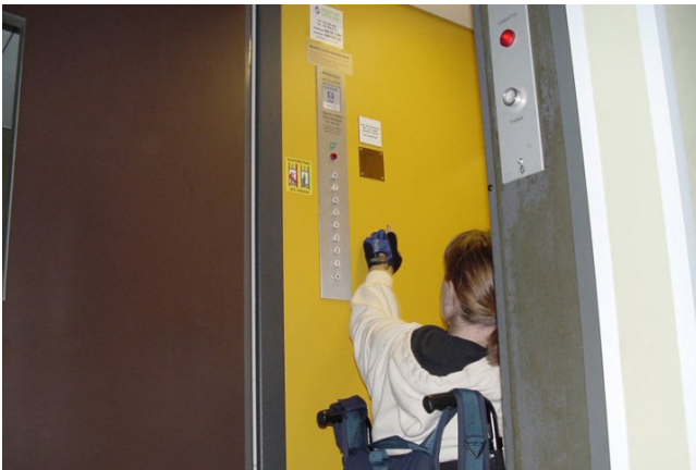
Fig. 72. Operating buttons difficult to reach. Vertically placed operating buttons are difficult to reach, especially for children, people of short stature and wheelchair users. It is recommended to place operating buttons in a horizontal row at a height of 900–1100 mm.
