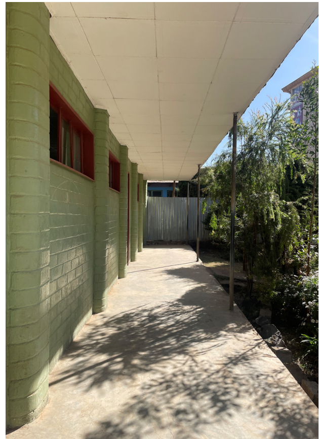
Fig. 77. Lack of protective elements. This outdoor hallway lacks protective elements on its right side, creating a potential falling risk. It is recommended to install a handrail or other protective element to ensure safety.
