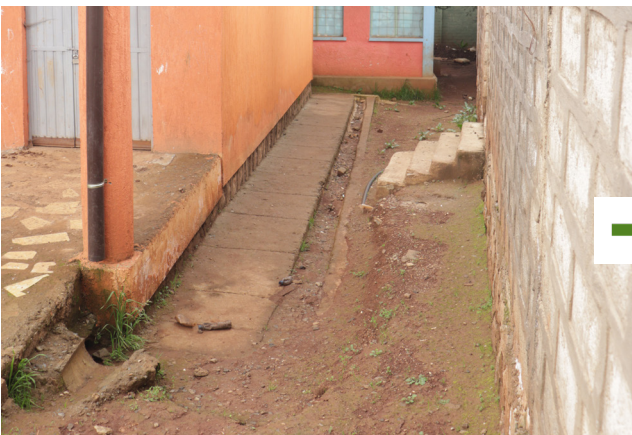
Fig. 8. Pathways (before). The pathways presented various accessibility challenges due to uneven surfaces and open gutters along the routes.
